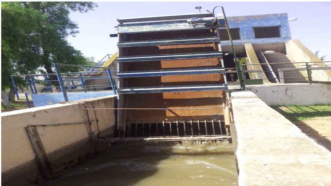
Figure II.3: Grille grossière manuelle (1unité).
