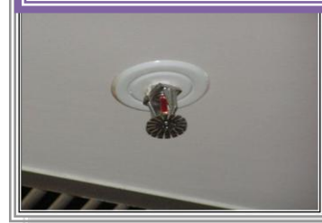
Figure 206: Illustration de Sprinklers
