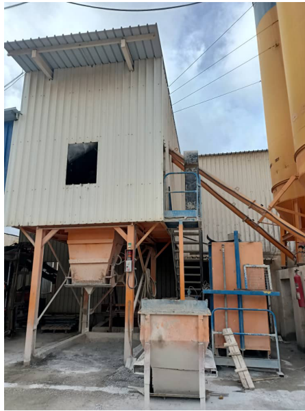
Figure 1.6: Concrete batching plant
