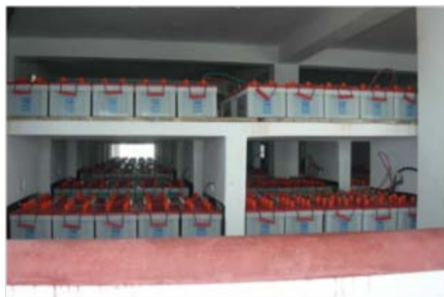
Fig. 8: Battery bank of 1000 kW capacity WBHPP at Kutubdia Island, Cox's Bazar.
