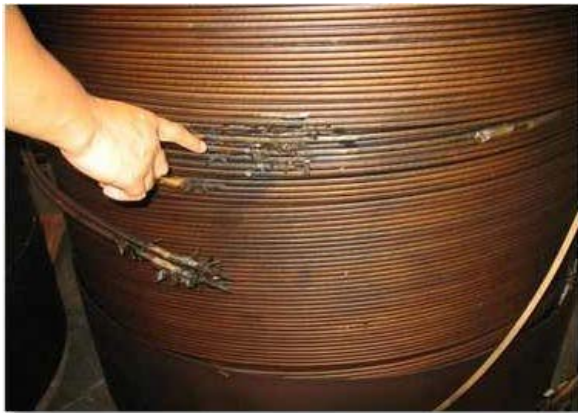
Figure 10 : Damaged LV (phase-C) coil
