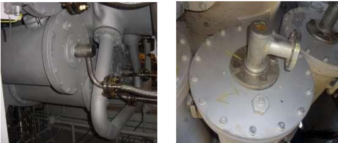
Figure III.11. Buses de carburant.
