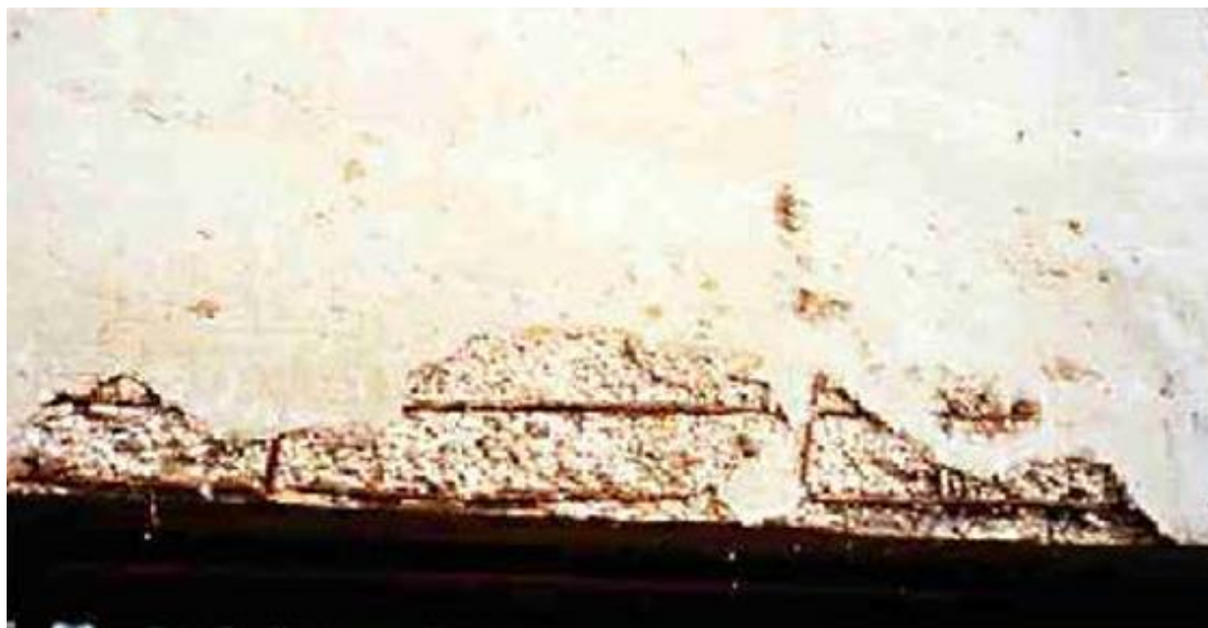
Figure II- 3:Corrosions des armatures
