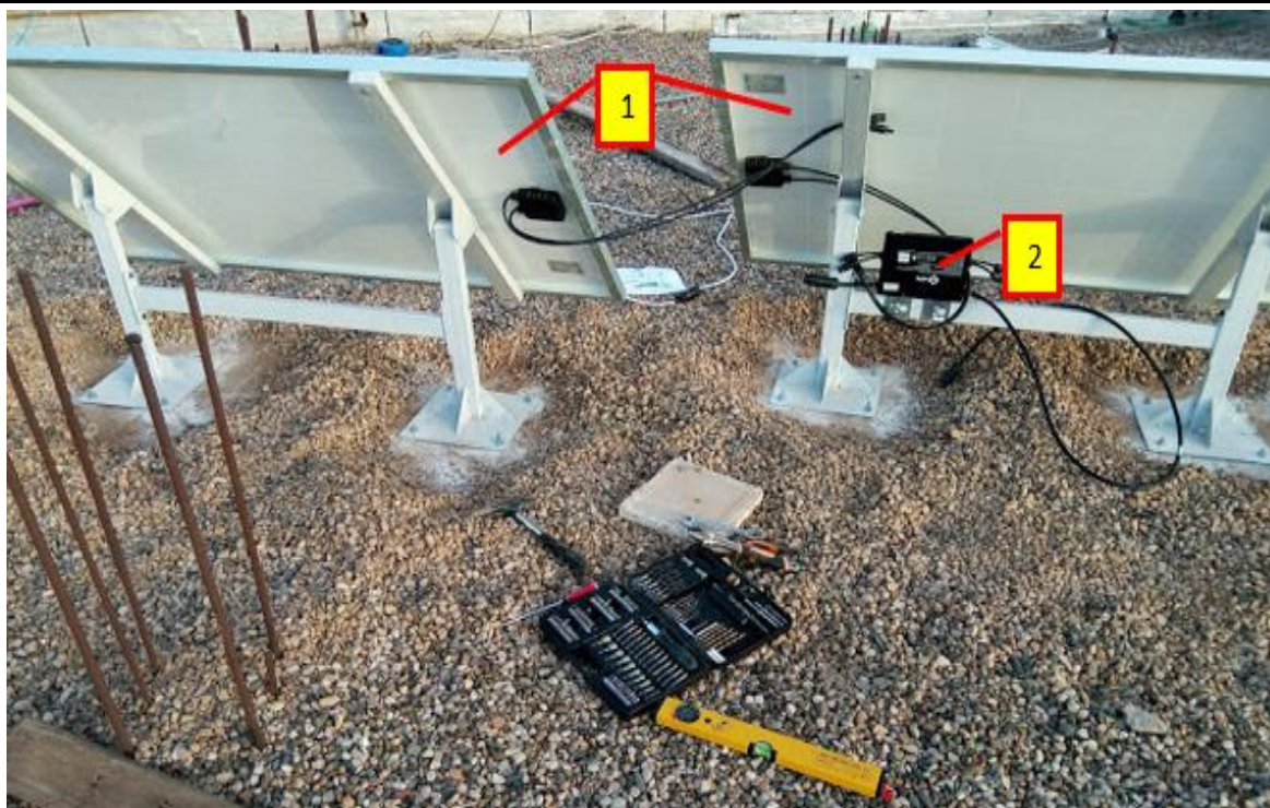
Figure 6.16 Experimental hardware setup of the PV industrial MP
