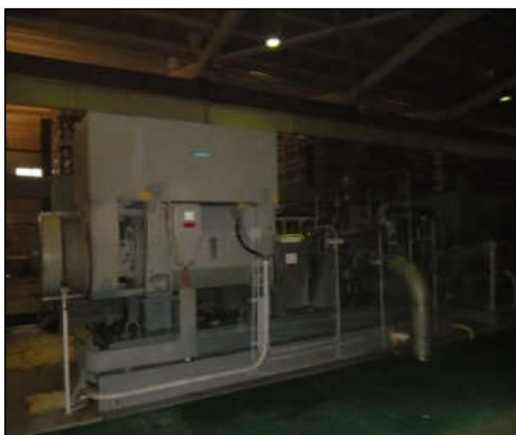
Figure 18 : Pompe Haute Pression (HP)
