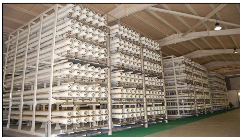
Figure 17: Unité d'osmose inverse (racks).
