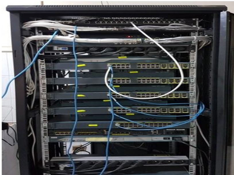
Figure IV-1 le Rack de ICT-TOWERS
