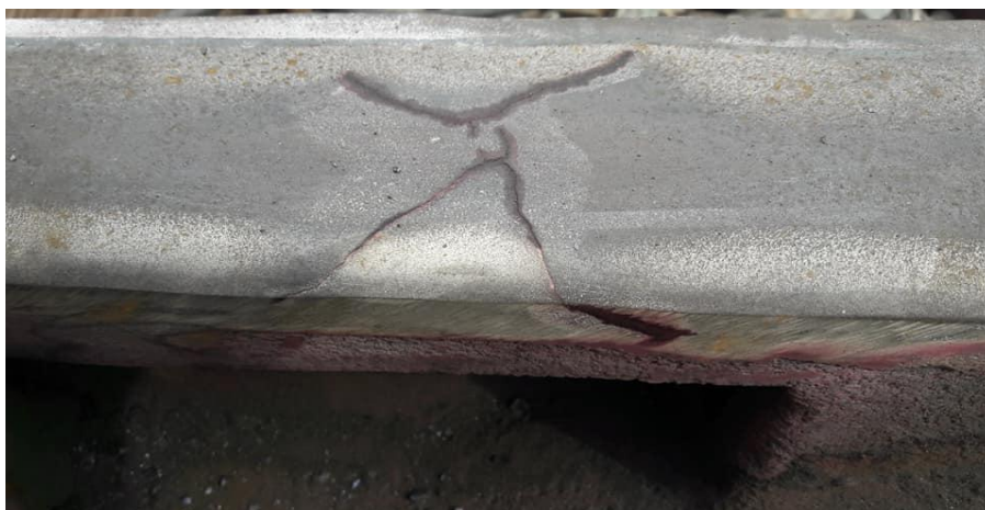
Figure II 3: Fissure sur rail [11]
