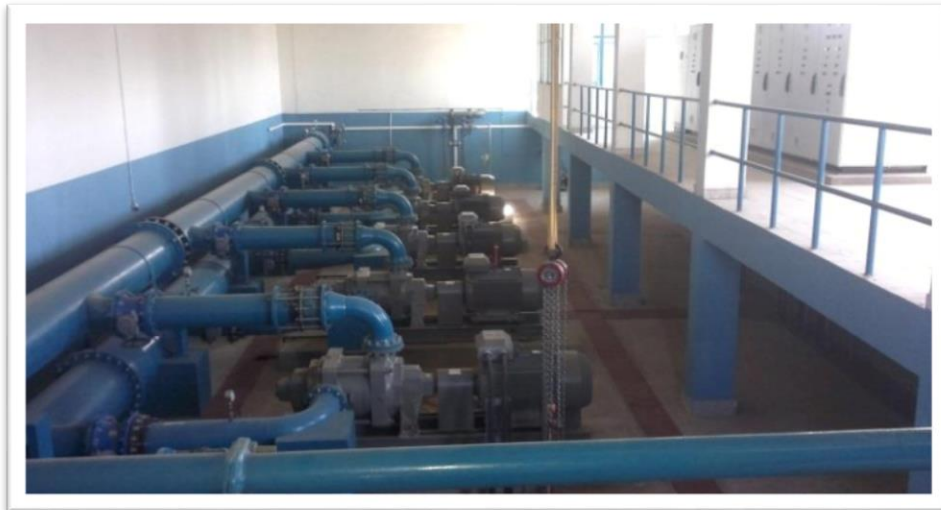
Figure 01 : Station de pompage [6]
