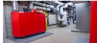
Figure 22 : chaudières gaz, source : https://remeha.be/wp-content/uploads/2019/04/project_sportingenkpark_04.jpg
