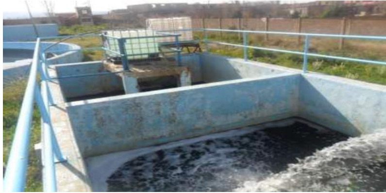
Figure (II.12) : Poste de chloration.
