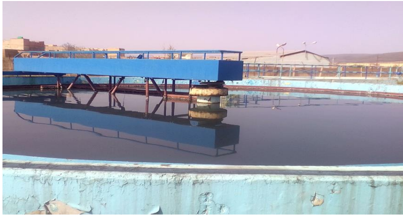
Figure (II.11) : Bassin de clarification finale.
