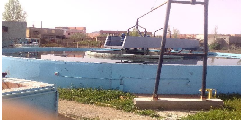
Figure (II.6) : Flocculateur – Clarificateur.
