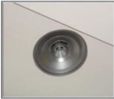
Figure 108:bouches de soufflage
