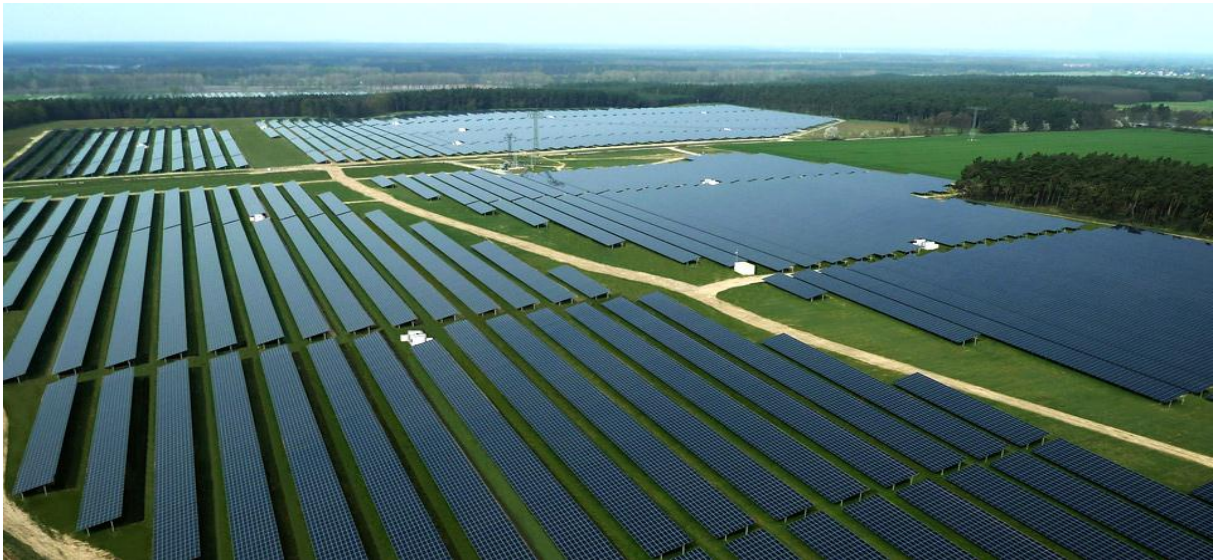
Figure (A. 4) Centrale photovoltaïque [18]
