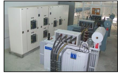
Figure 132: poste de transformation
