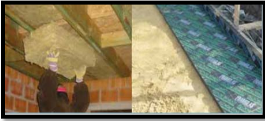
Figure 52: isolation des planchers
