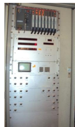
Figure 2.8. Tableau PLC – ELBO
