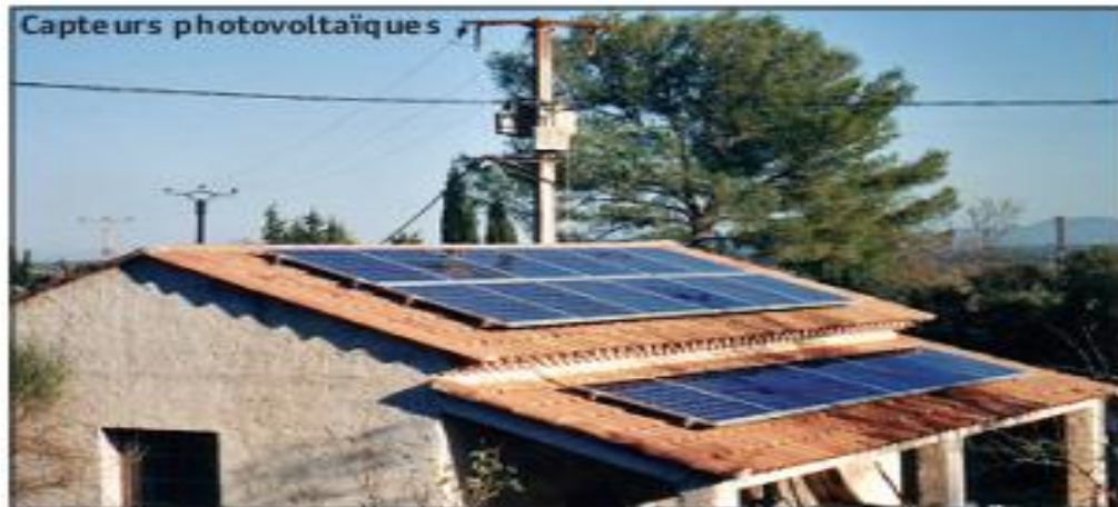
Figure (II.18) Capteur photovoltaïques [21]
