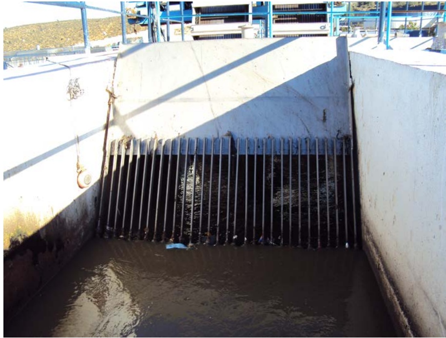
Figure III. 10: Grille grossière manuelle
