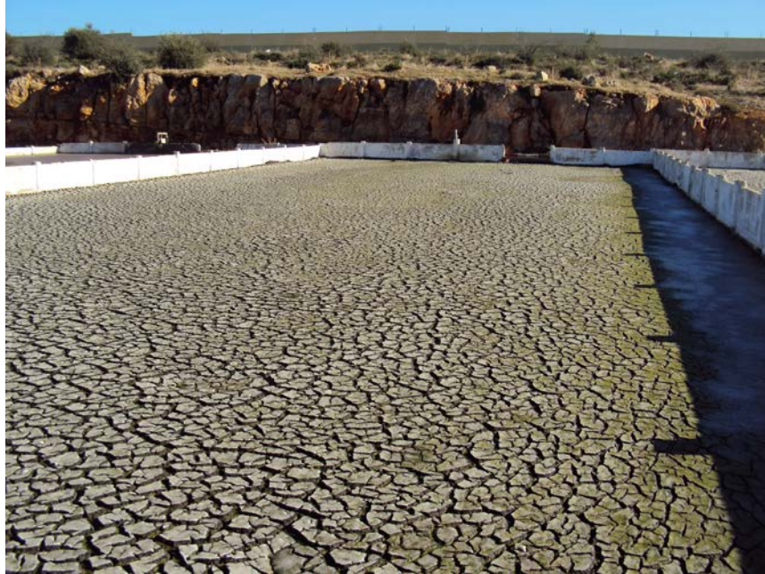
Figure III. 17: Lits de séchage
