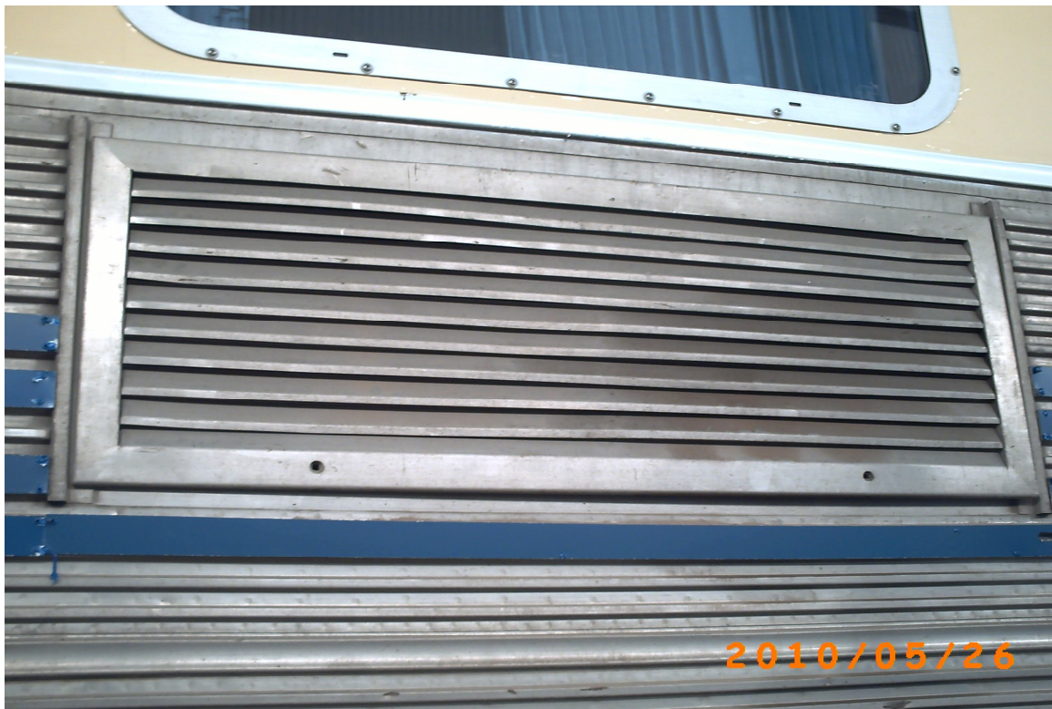
Figure (I.1): Gaine de reprise.
