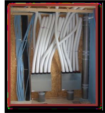
Figure III.90: Les gaines techniques
