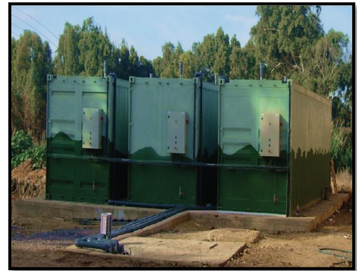
Figure 27: station de traitement des eaux usée "oxybatch"
