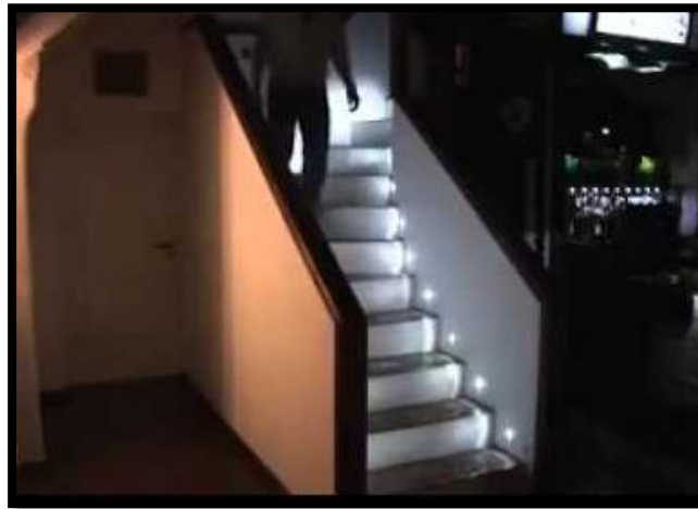
Figure 95 : Eclairage LED automatique 114
