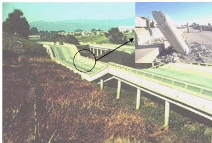
Figure 1.8 Effondrement du pont route 1, Struve Slough, Watsonville. (1989) [1]
