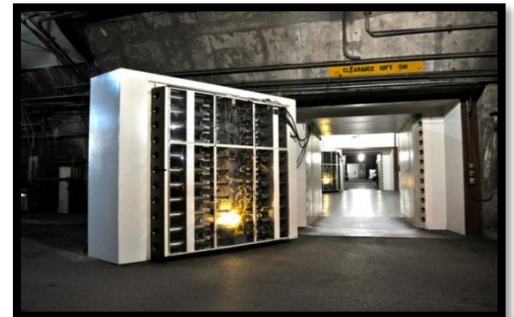
photo 46 : Porte anti souffle https://en.wikipedia.org/wiki/Cheyenne_Mountain_Complex#/media/File:NORADBlast-Doors.jpg
